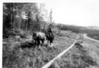
#121: Where is this? The road is finished and the fuel pipeline to the airfields lies on the ground under the open-wire telephone lines.
